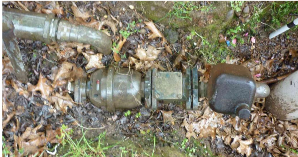
Figure 1: The Main Water Meter at Bright Chalet
